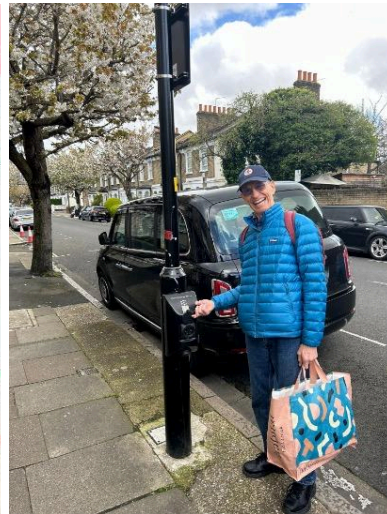
London Light Pole Charging
