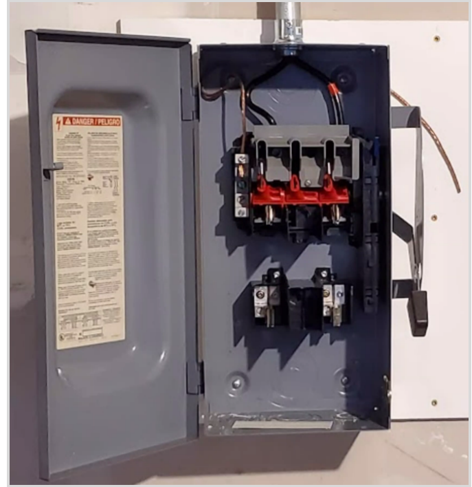
Square D shutoff switch and fuse disconnect panel provides added protection (just in case!) up to 20k volts DC shorts and tries to flow from the car battery back to the AC wiring in the house. Also a convenient way to turn off power to the charging system from the garage if needed
