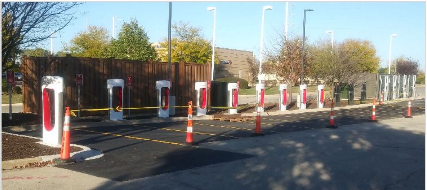
Tesla chargers being installed at the North end of the Meijer parking lot on Rt. 59 Naperville
