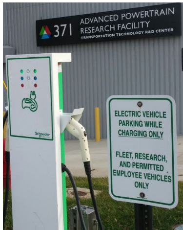
EVSE in use at the lab
